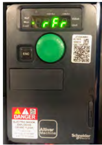
OUTPUT FREQUENCY DEFAULT SETTING OF VFD INDICATES MOTOR FREQ.
