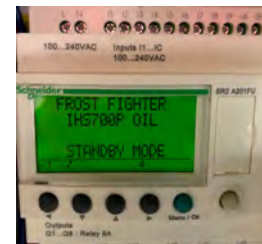
PLC DISPLAY BEHIND MAIN CONTROL BOX COVER.
