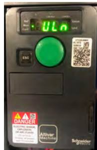
MAINS VOLTAGE VOLTAGE FROM DC BUS.
