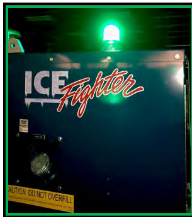
Beacon Displays Steady Green when Generator is Operating and Supplying 120VAC
