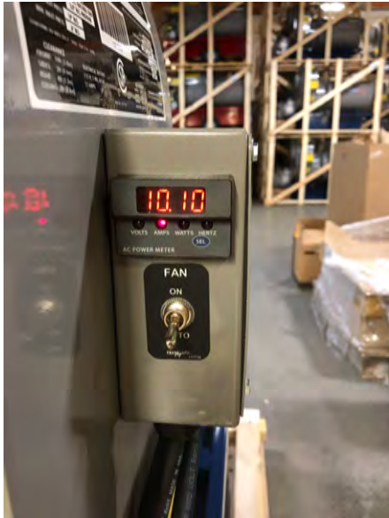
Meter showing total amperage draw for the unit
