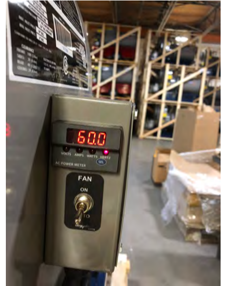
Meter showing the hertz being supplied to the heater
