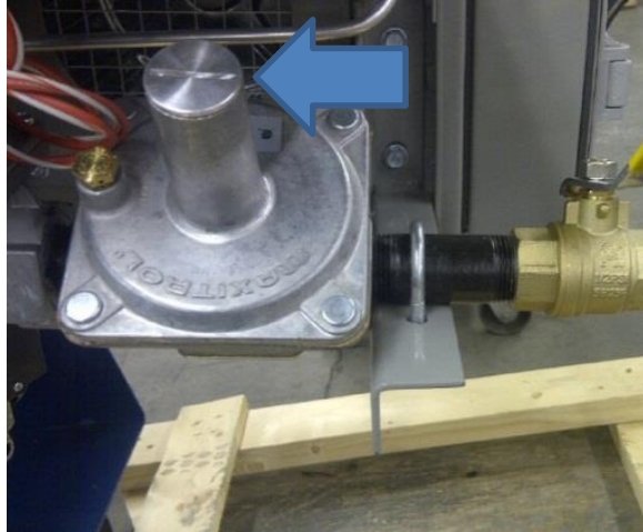
Figure 3: Regulator top cap location
